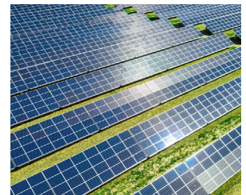
Solar Plus Battery Energy Storage Microgrid - Most feasible on Salt Cay and North Caicos based on land availability, energy demand, infrastructure and other key factors
